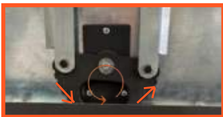
Close Damper Control
